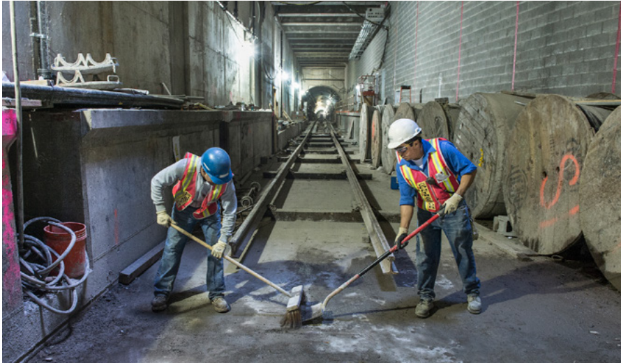
Photo: Metropolitan Transportation Authority/Patrick Cashin. Men working in a subway station construction, New York, USA, 2014 < https://goo.gl/BkKdhZ >.
